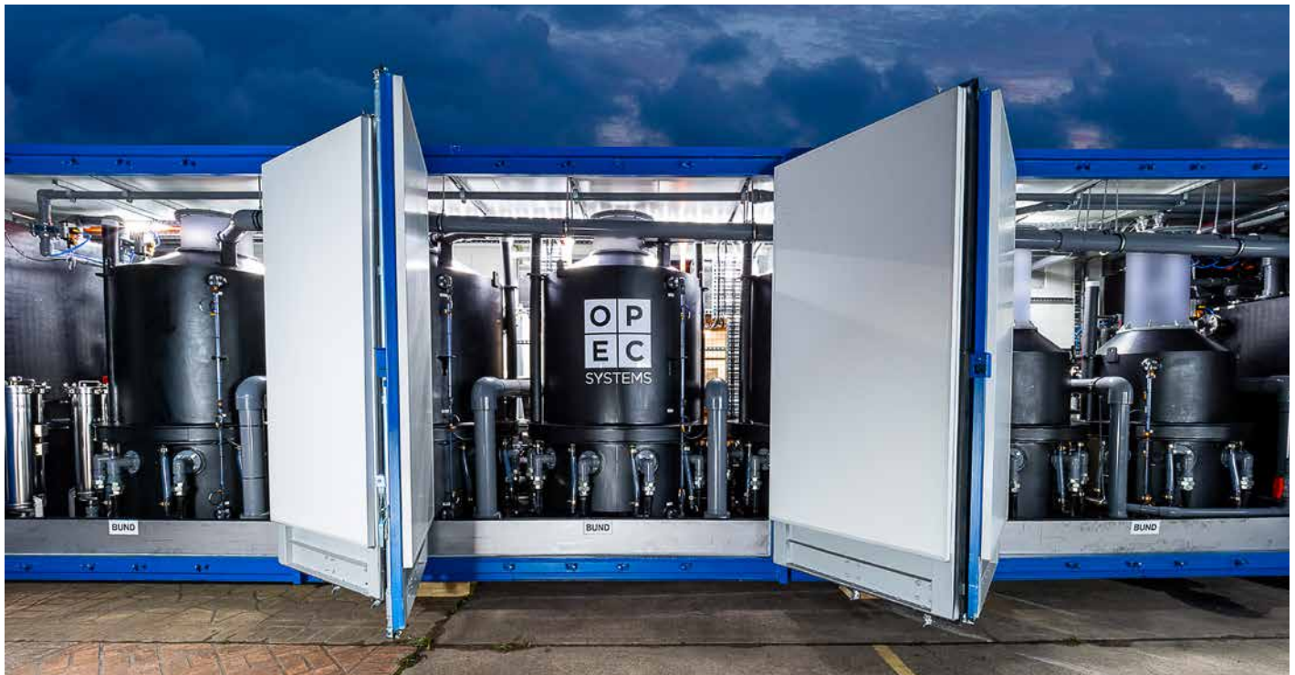
Figure 4: Photo of a SAFF40 treatment plant
