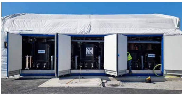
Figure 1: Full scale SAFF40 treatment system installed at Tveta Landfill
